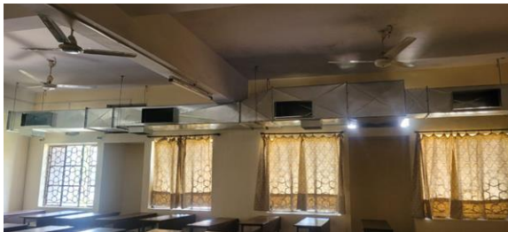
Figure 1: Setup of Duct Air Cooler in Classroom
