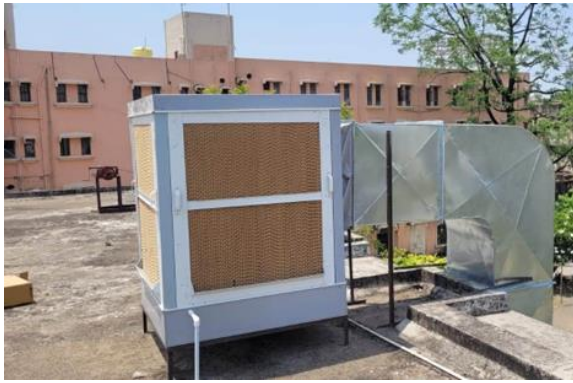
Figure 1: Setup of Duct Air Cooler
