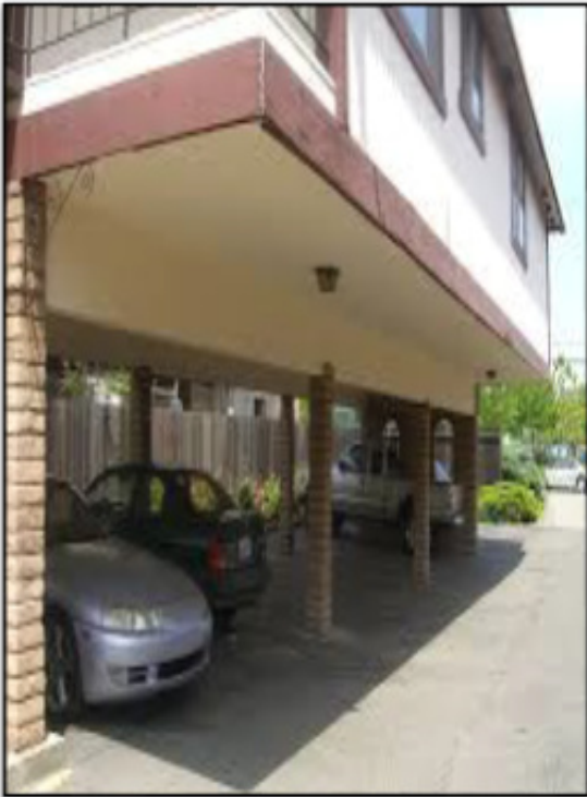
Figure 1: Soft Story for Parking Floor
